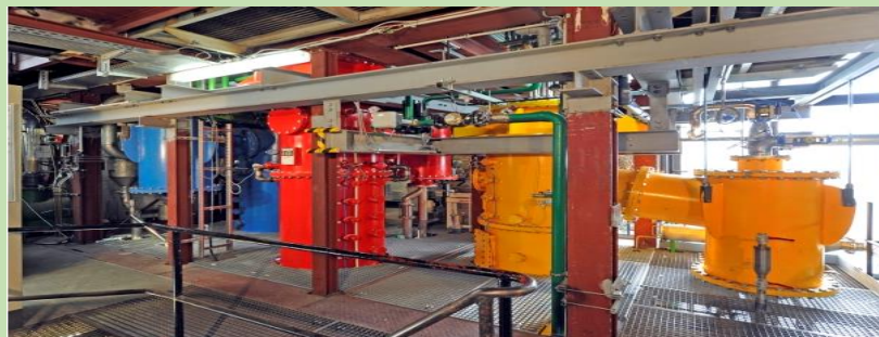
Alstom Power Calcium Looping – TRL 3
